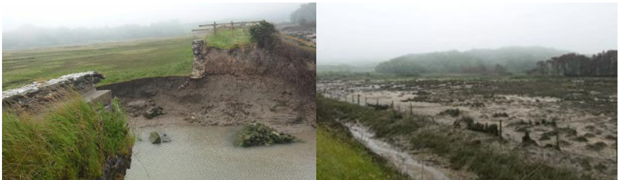
Left to right: Seawall breach. Saltmarsh development on landward side (right)
